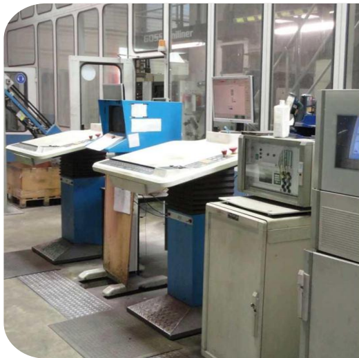
Existing control system to be replaced...
